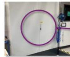
Main control cabinet
